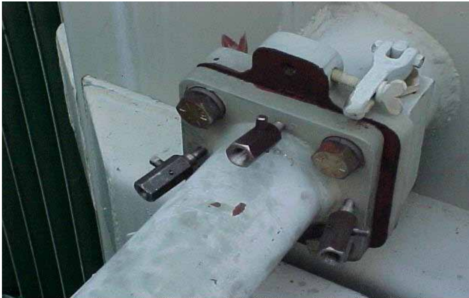
A Flapper Valve Flange That Has Been Drilled & Tapped - Ready For Injection
