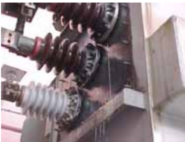
Leaking Bushing Flange prior to the Clamp Installation
