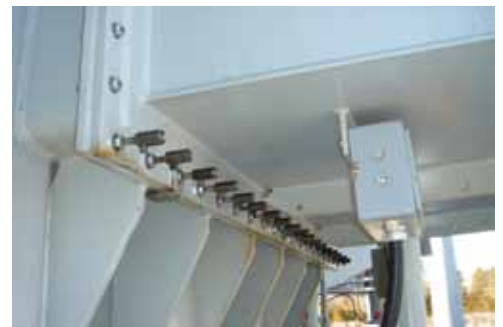
Tap changer flange ready to be sealed.
